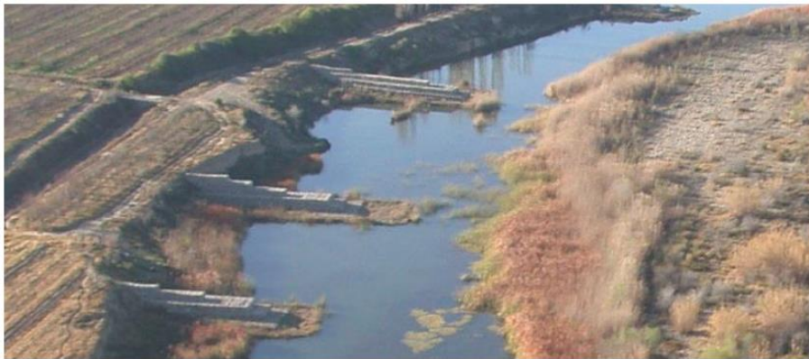
Figure 1.1 Spur dike protects a bend in the Gamka River at Calitzdorp, South Africa (King, 2009)
