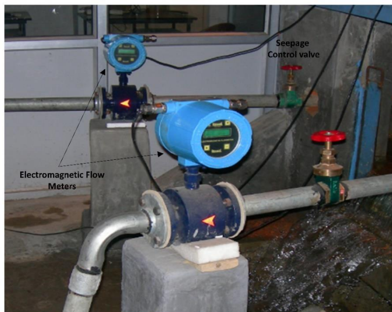
Figure 2.6 Electromagnetic flow meters for seepage discharge measurements
