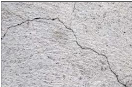
c) Cracks in slab due to thermal stress
