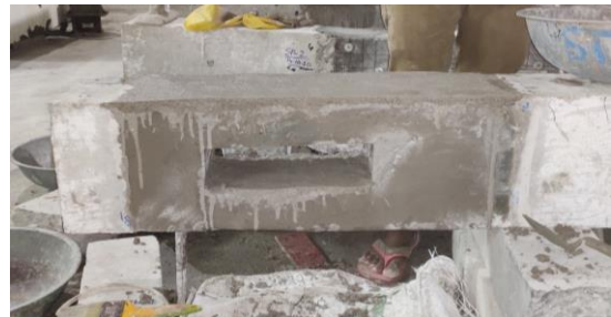
g) Repaired beam with opening in shear Zone
