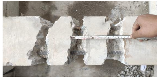
b) Widened cracks
