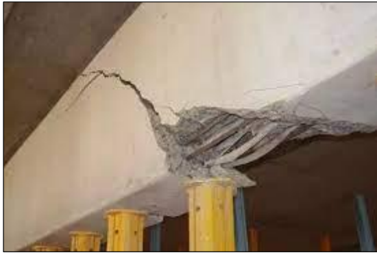
a) Failure of beam due to over loading
