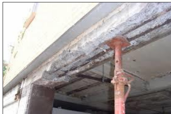
d) Cracks in beam due to corrosion in steel
