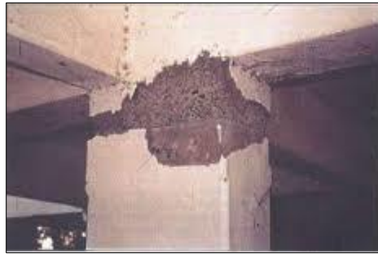
b) Cracks in column
