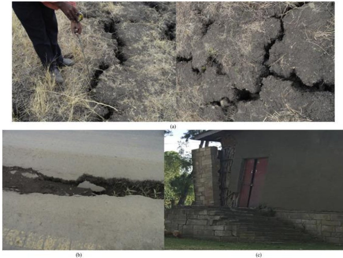
Fig.2.5. Typical cracks in black soils during the dry season: (a) field condition; (b) pavements; (c) buildings (Atahu et al. 2019).
