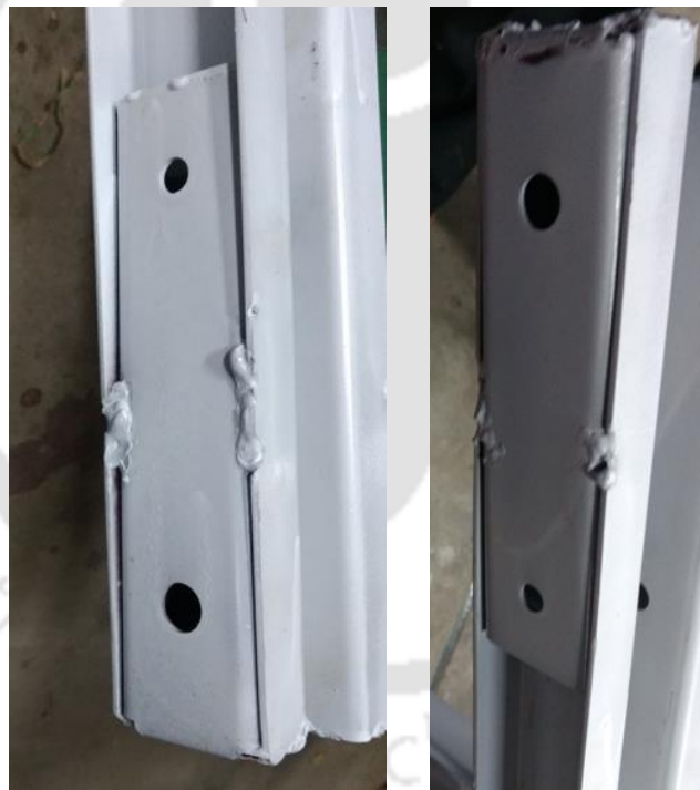
Figure 4.90: Joining and Welding defect
