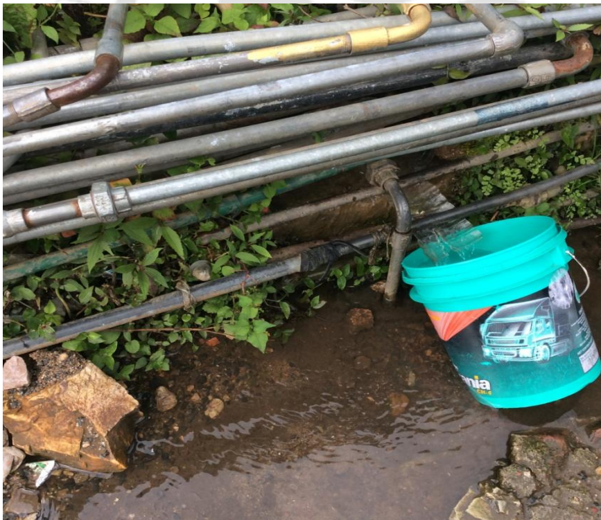
Plate 2.1: Leaked Pipes in Mawprem ‘A means of accessing of water for the poor’!
