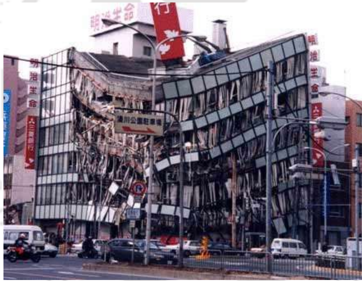
Figure 1.1 Collapse of steel building during January 17, 1995, Kobe earthquake, Japan (Elkholy S & Meguro K (2004))
