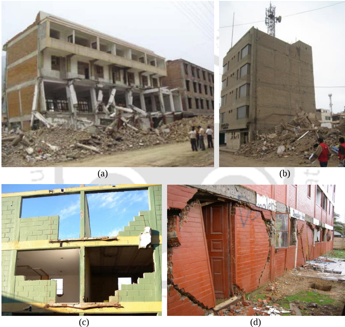
Figure 1.3: Performance of CM buildings during past earthquakes: (a) Severely damaged RC building adjacent to undamaged CM building in 2008 Wenchuan, China earthquake (Wang 2008), (b) Undamaged six-story CM building adjacent to collapsed URM building in 2007 Pisco, Peru earthquake (Brzev and Mitra 2018), (c) Absence of RC tie-columns in walls with openings resulted in damage to CM building in the 2010 Chile earthquake (Brzev and Mitra 2018), and (d) damaged to the ground floor of a medium-rise CM apartment buildings in the 2010 Maule, Chile, earthquake (Brzev and Mitra 2018).
